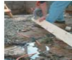
What are the hazards shown in these photos?
