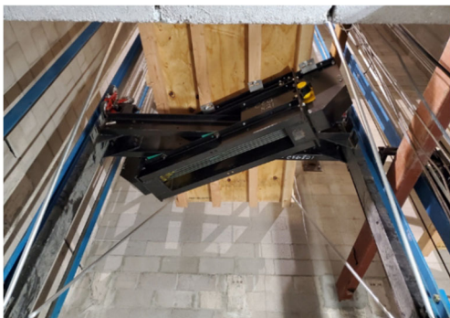
Elevator with overhead protection canopy
