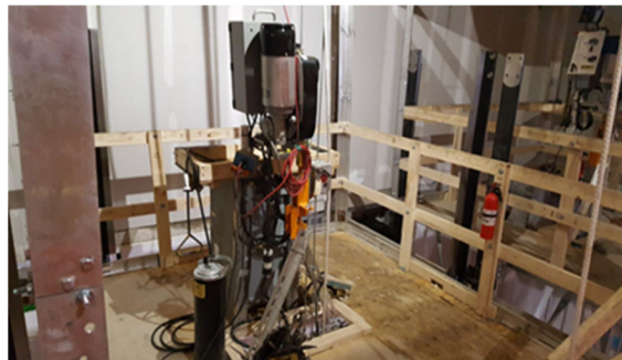
Temporary hoist machine attached to a false car
